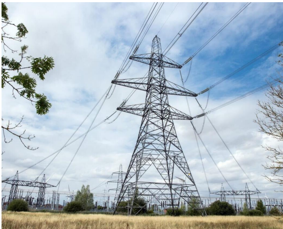
Image 5.13 Typical terminal lattice pylon 3
